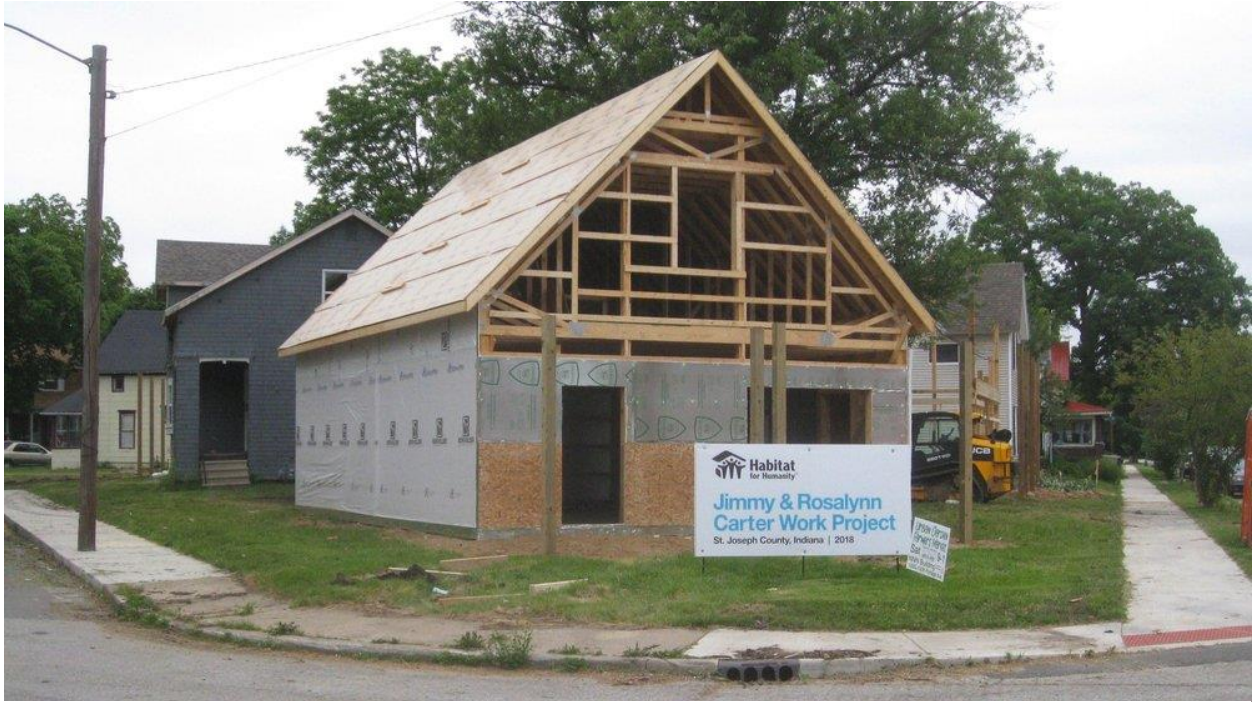
A net zero home project in South Bend, IN, by small-scale developer Mike Keen, in collaboration with Habitat for Humanity.
